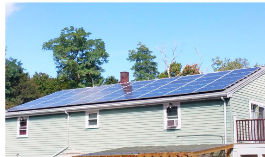
12.3 kW system installed by USA in Avon, MA
