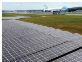
DOT/FAA, Chattanooga Airport, 3MW
