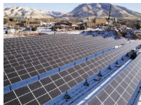
VA Hospital, Salt Lake City, 600kW, ground mount
