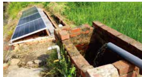
PV Water Pumping System
