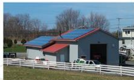
16 Kilowatt steel roof mounted system
